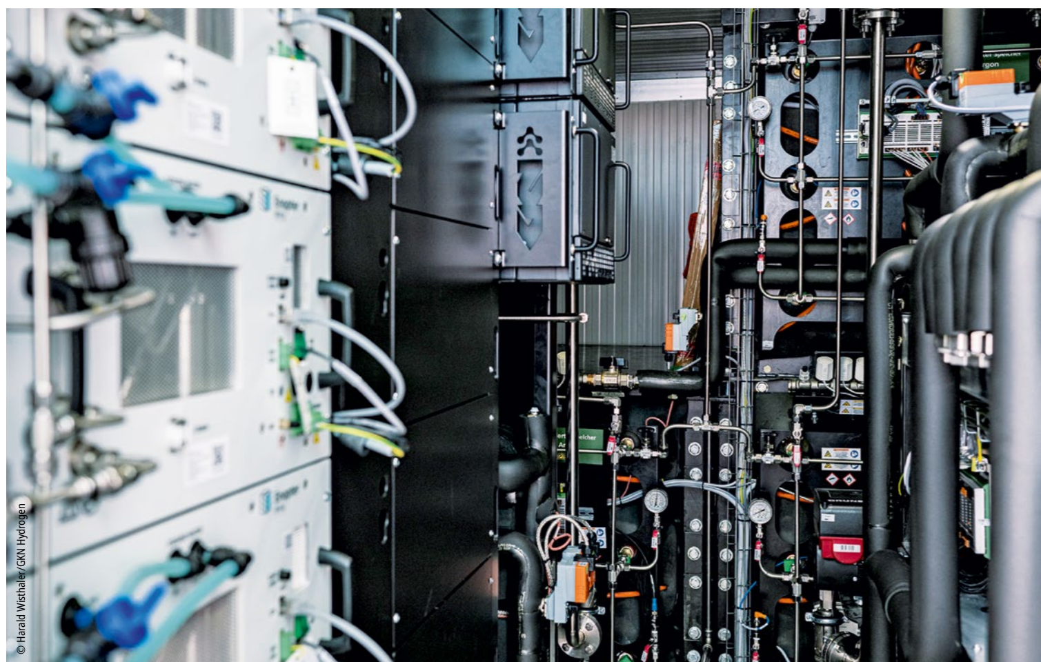
The sophisticated inner workings and associated diverse process sequences require flexible, scalable, and reliable control technology.
