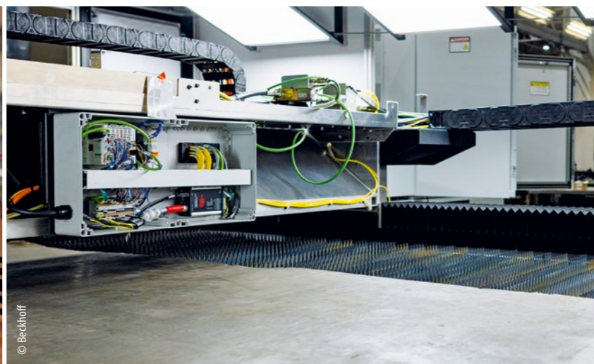
View into the CLX Fiber Laser System with several EtherCAT Terminals installed in a decentral switch box
