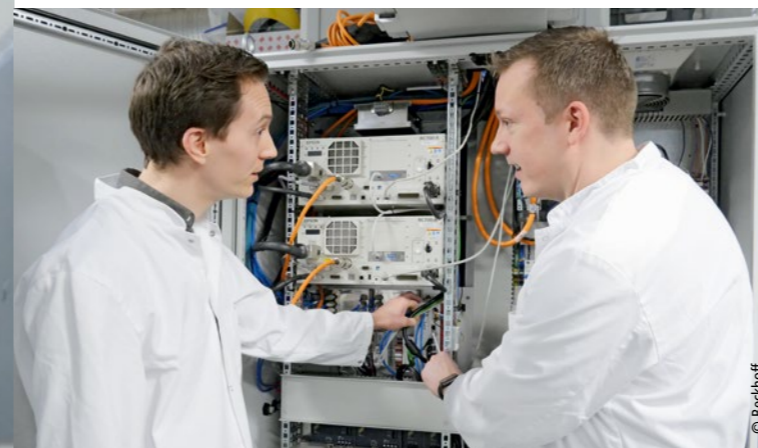
Rune Callesen (left), head of the automation department at Elos Medtech, and Rasmus Jensen (right), support engineer at Beckhoff Denmark, in front of the control cabinet of the blister packaging machine that will also provide carton packaging in the future.
