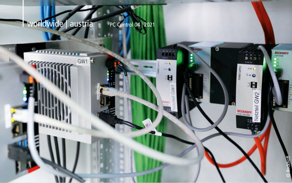
Ultra-compact C6030 Industrial PCs (left) – supplied via Beckhoff PS series power supplies (right) – play a central role as edge gateways.
