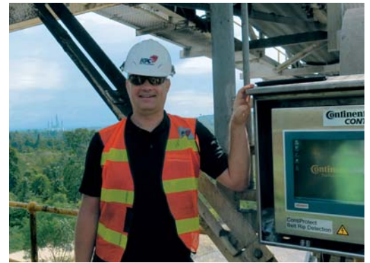
On site in Borneo: Hans Christian Enders, Industrial Solutions division of Continental Engineering Services GmbH, next to the control cabinet of the BRD system.
